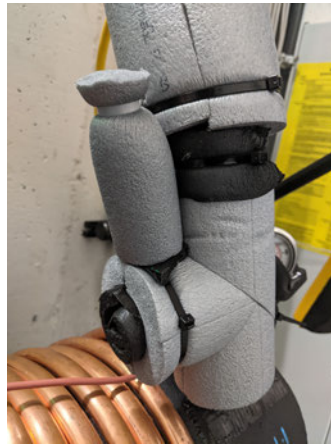
Figure 4.3: Insulation of the valves
