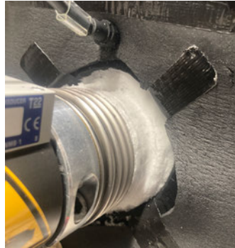
Figure 4.2: Ice around coupling and shaft
