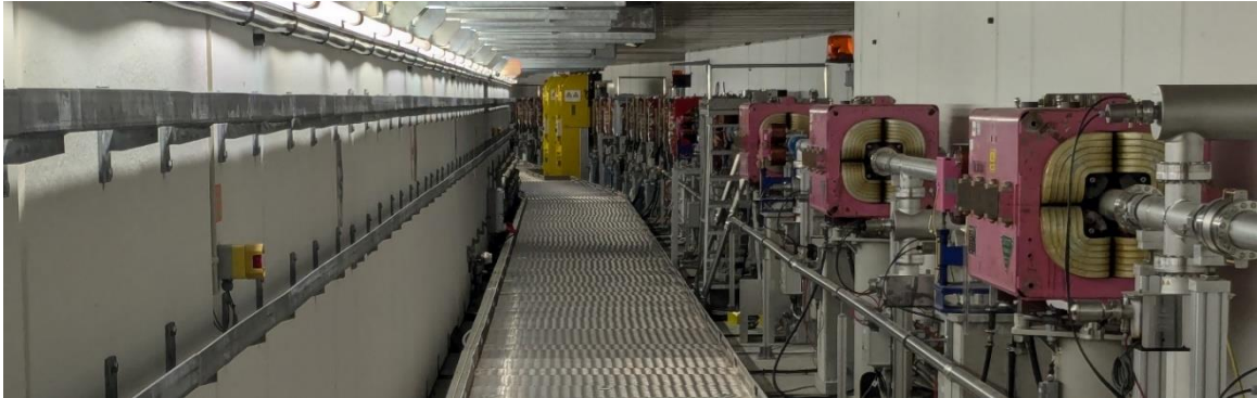
Figure 9: PETRA III tunnel (picture provided by Jonas Albers)
