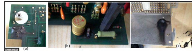
Figure 13: Photos of an energy compound of a mechanical ventilator. a) Electric platine from the bottom. The copper connections are burned. b) The electrode (middle) is burned, the capacitor next to the electrode is damaged and not functional anymore. c) The metal case of the electric platine. The force of the burning/explosion of the electrode can be seen.
