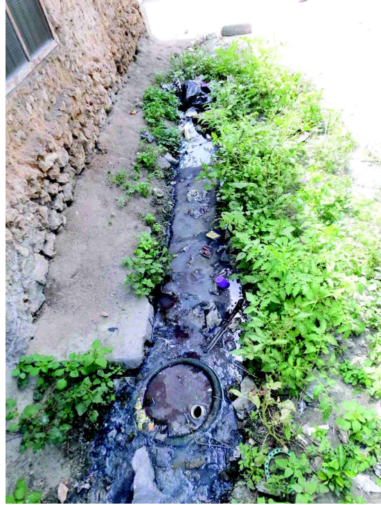
Stagnant water from domestic outflow
