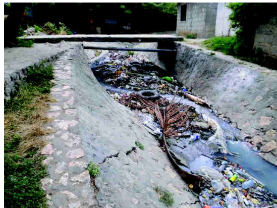
Waste disposal drainage - Shaurimoyo
