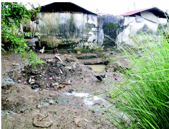
Burst drain during rain season
