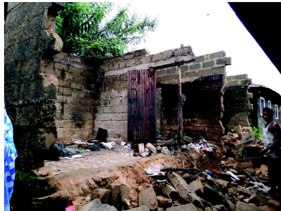
Collapsed house due to heavy rainfall
