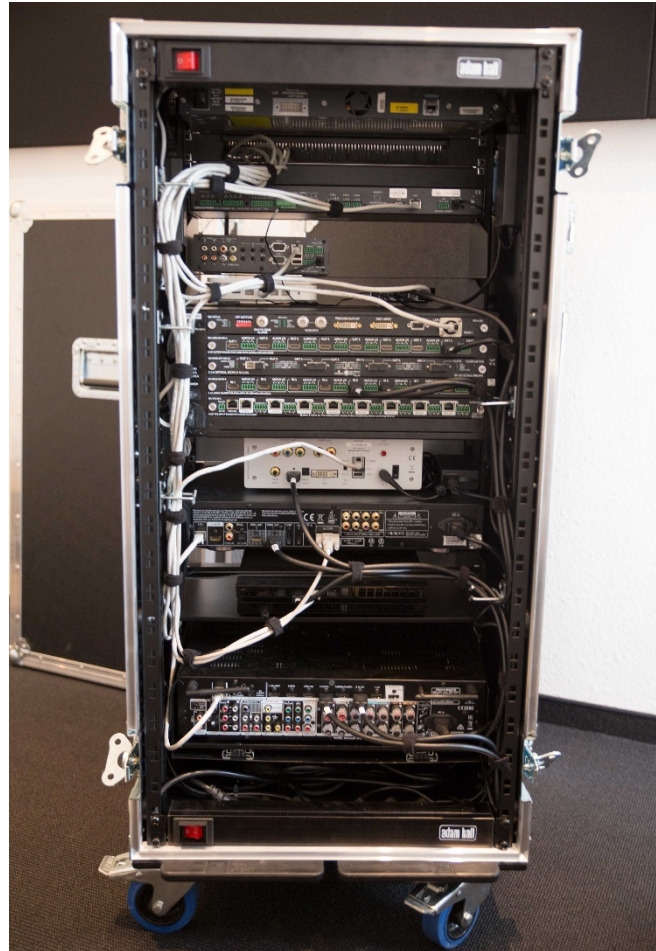
Figure 24: Final internal rack cabling
