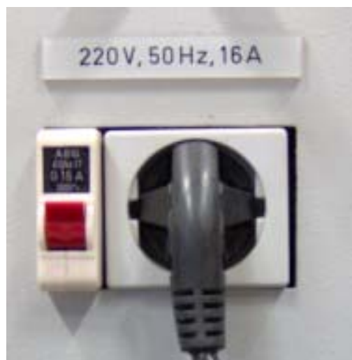
Figure 5.5 Power supply 220 V
