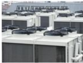
Climate control units
