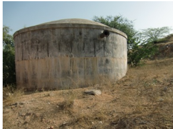
Figure 9: Main/ Central GLR Thoomba Ka Goliya located near sand dam. Image taken by the author 22.03.2017.
