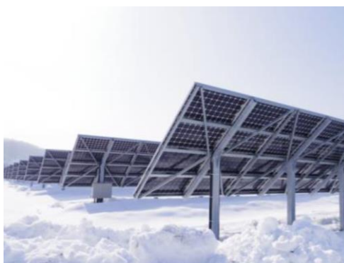
Figure 3.11 Large-scale power plant for fixed tilt angle, 1.25 MW, “Hokuto”, Japan, by PVG Solutions [Ish16].
