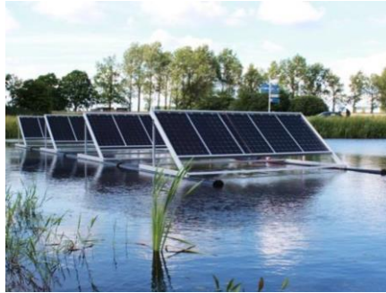
Figure 3.9 Pilot test of 5.5 kWp Bifacial PV system Sunfloat [Kre17].
