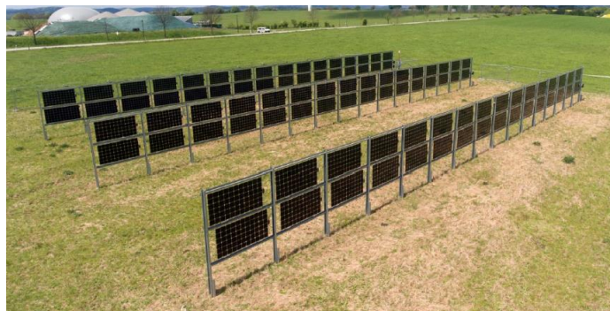
Figure 3.6 Pilot test of 28 kW vertical bifacial E-W oriented PV system in Saarland, Germany by Next2Sun [Hil17].
