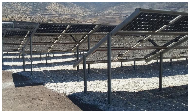
Figure 3.12 Large-scale power plant for fixed tilt angle, 2.5 MW, “La Hormiga”, Chile, by MegaCell Group [Kop18]
