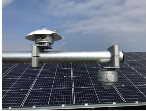
Figure 6.12. Set up for the albedo measurement from Hukseflux, composed of two pyranometers; one facing the sky and the other facing the ground.
