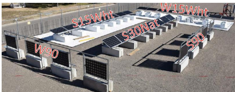
Figure 3.2 Photograph showing the setup of monofacial and bifacial modules installed at the Prism Solar test, in Albuquerque [Ste17].
